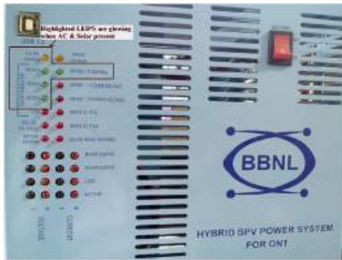
Fig. 3.12.9. Highlighted LED's are glowing when AC & Solar Present
