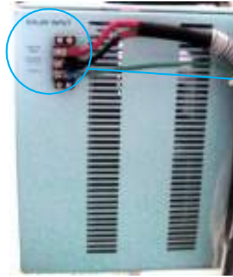
Fig. 3.6.7 Solar Panel CCU Connectivity
