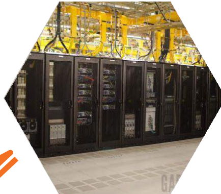
Fig. 1.2.8 Mobile Switching Centre
