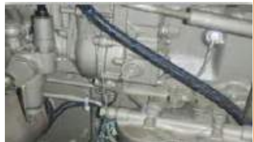
Fig. 2.9.9(iii) Fuel flowing out from Air Vent
