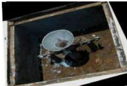
Fig. 2.4.4(ii) Internal View of Earth Pit Chamber
