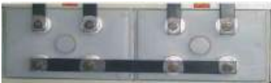
Fig. 2.2.16(i) Clean the batteries as and when dust accumulates
