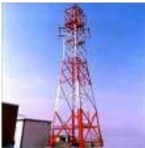
1. Tower for installing BTS and Micro Wave Radios.
