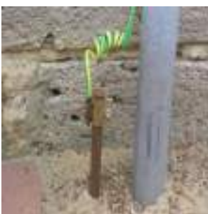
4. Earthpit for providing controlled Earth at site.
