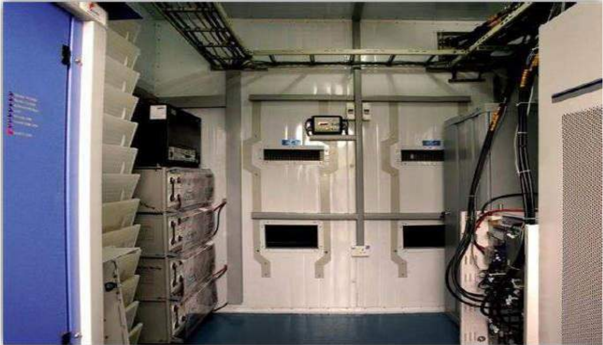
Fig. 2.1.11(i) Typical View of Equipments Inside the Telecom Shelter
