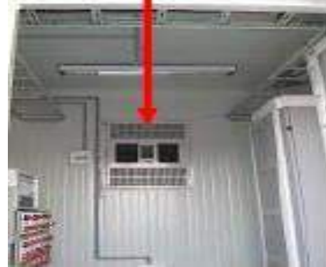
Fig. 2.7.2 Air conditioning in a Shelter
