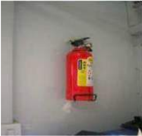
Fig. 2.3.4(i) Fire Extinguishers
