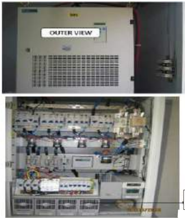
Fig. 2.2.21 Inner and Outer of a Power plant
