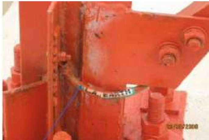
Fig. 2.5.1(iii) Earthing of a Lightning Arrester
