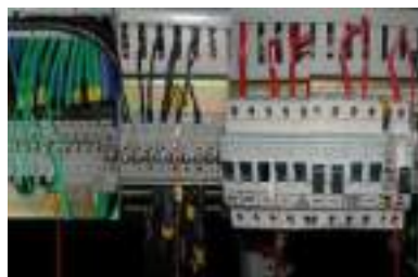
Fig. 2.2.2(vi) Ac Distribution Panel
