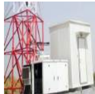
3. Shelter Room is used to Provide space for equipment.
