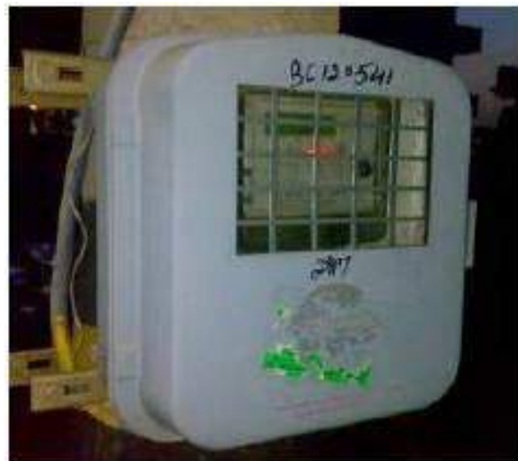
Fig. 2.4.1(ii) Electricity Meter to measure the power consumed
