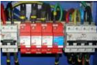
Fig. 2.2.2(ii) Lighting and Surge Protector
