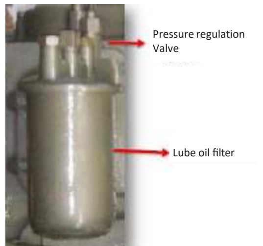
Fig. 2.5.7(viii) Oil Filter and Pressure Regulation Wall
