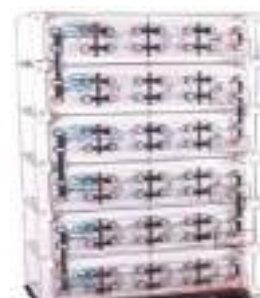
6. battery Bank Power Storage is used as backup power when there is no input power at site.
