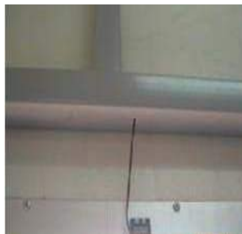
Fig 2.3.4(iv) DOOR CLOSE SENSOR: Generates alarm if the shelter door is open
