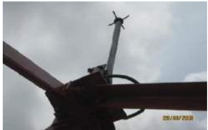
Fig. 2.5.1(ii) Installed Lightning Arrestor at a Tower Top
