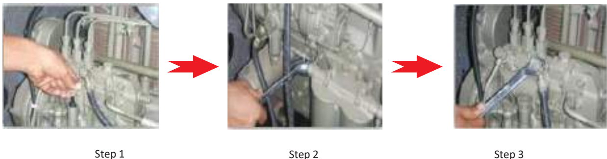
Fig. 2.9.9(i) Bleeding of DG Set
